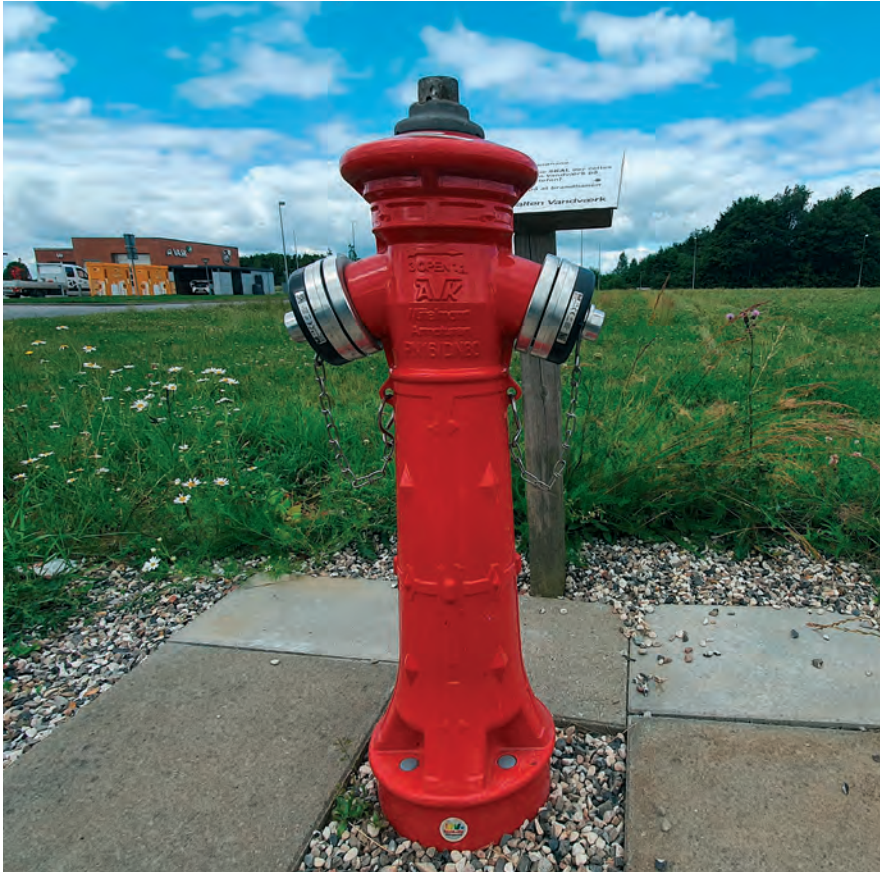
Hydrant with VIDI Caps installed. The use of a hydrant affects the pressure in an area. Therefore, it is important for the utility to know when the hydrant is being used in order to distinguish between a pressure drop coming from regular use or from a pipe burst.
